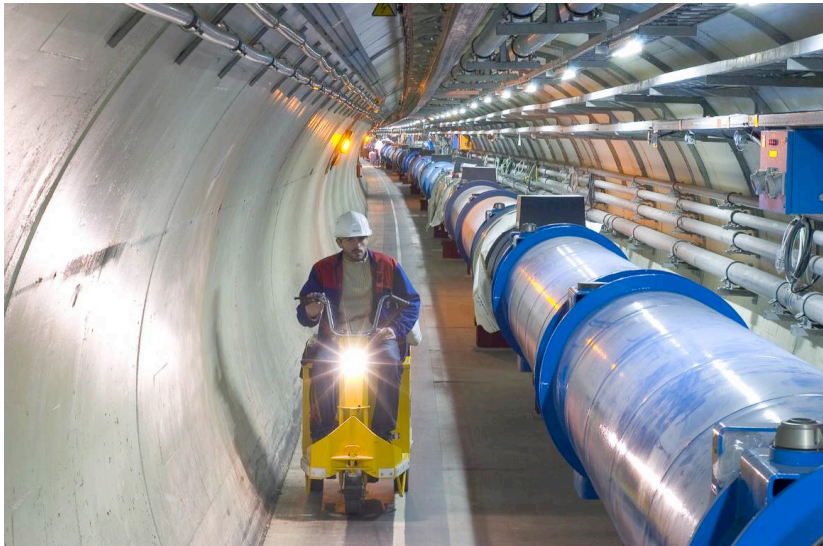
LHC tunnel: a long periodic lattice of superconducting 80 kGs (8T) magnets
